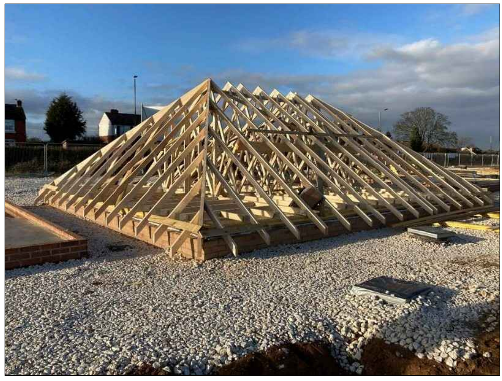
GENERALLY SCAFFOLD BUILT AROUND ROOF CONSTRUCTED ON GROUND. HOP-UPS TO BE LEFT OFF UNTIL ROOF LIFTED OUT ON DAY OF KIT ERECT.
